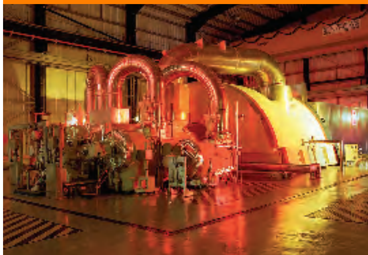
Turbine hall, Deeside, UK
