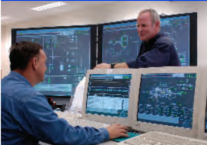
Control centre, Pelican Point, Australia
